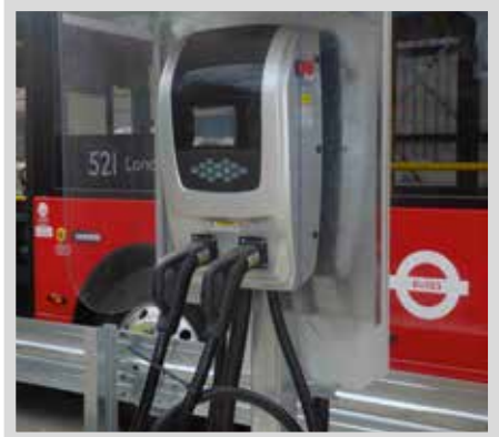
Charging point: One of 34 charging points for the new electric bus fleet.
